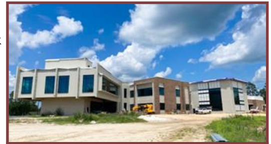
Recent photo of progress at the AMC facility, which will foster modern industrial practices, advancing new technologies and providing grounds for training the future manufacturing workforce with a focus on chemical and material manufacturing. Photo provided by B.L. Harbert.
