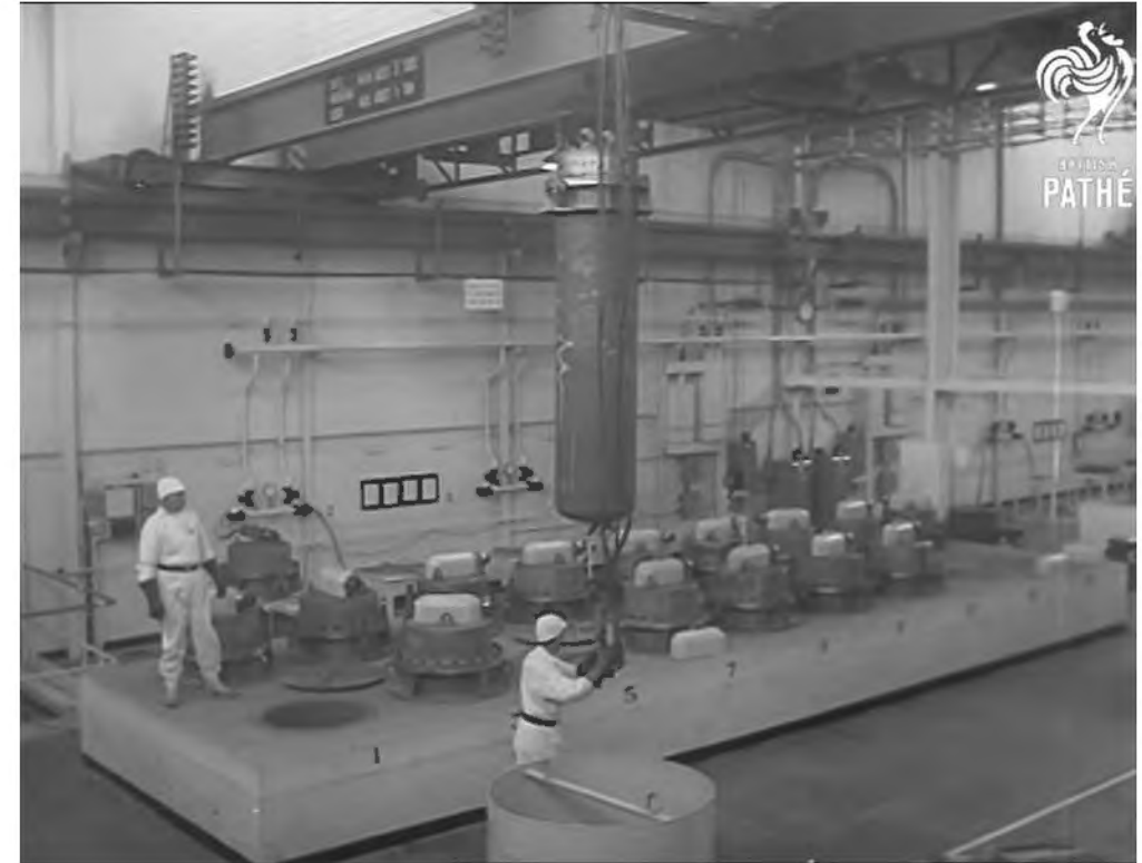
Metal Reduction Reactor Cool-Down Pens at Westinghouse's Springfields facility, circa 1959
