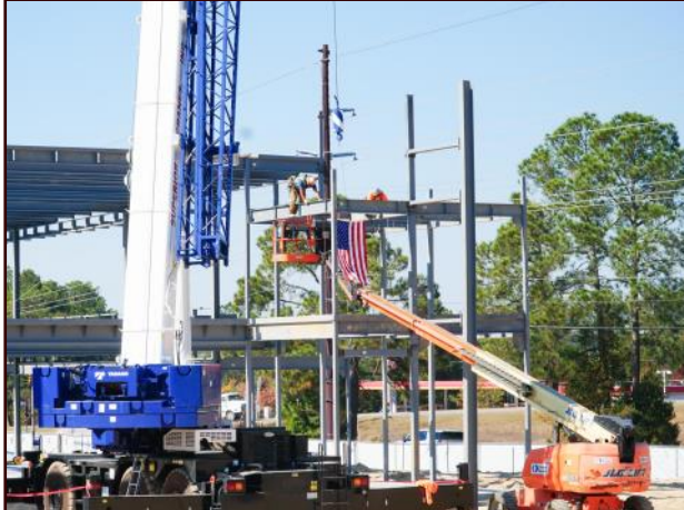
A construction crew lowers the last piece of structural steel into place on the Advanced Manufacturing Collaborative facility. Credit: DOE Office of Environmental Management Newsletter
