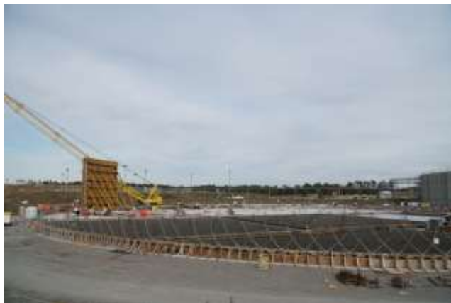
The first wall section of Saltstone Disposal Unit 8 is being constructed at the Savannah River Site.
