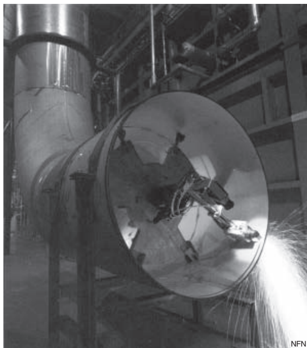
Figure 4. The Elbow Cutting Pipe Crawler was used to cut piping located 265 feet
